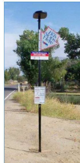
FIGURE 26: SOLAR-POWERED BUS STOP LIGHT.
