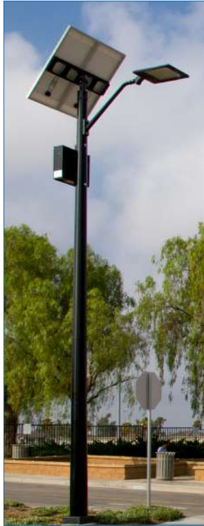
FIGURE 25: EXAMPLE SOLAR POWERED LIGHT
